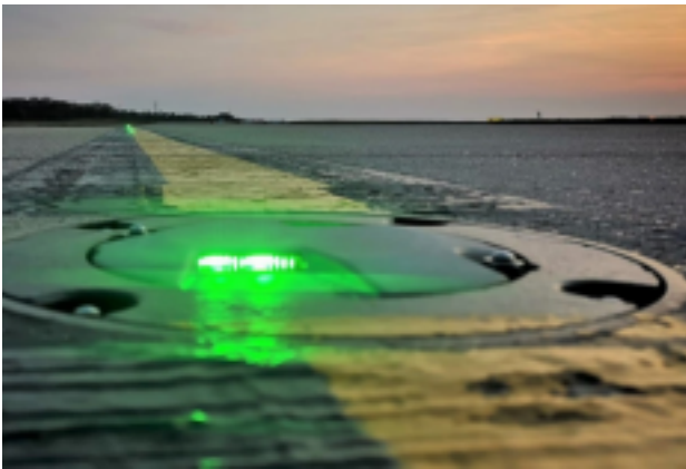
TKH Airport Solution
