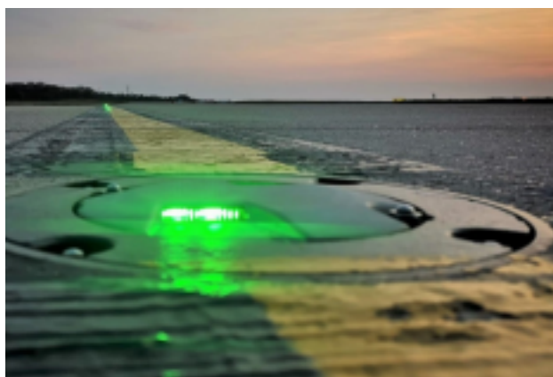
TKH Airport Solution
