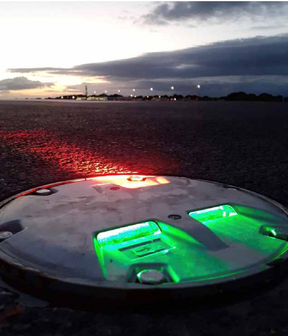
OCEM airfield lighting
